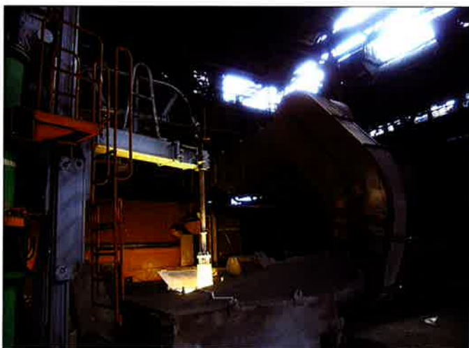
Fig. 5: Induction furnace during the melt bath injection process
